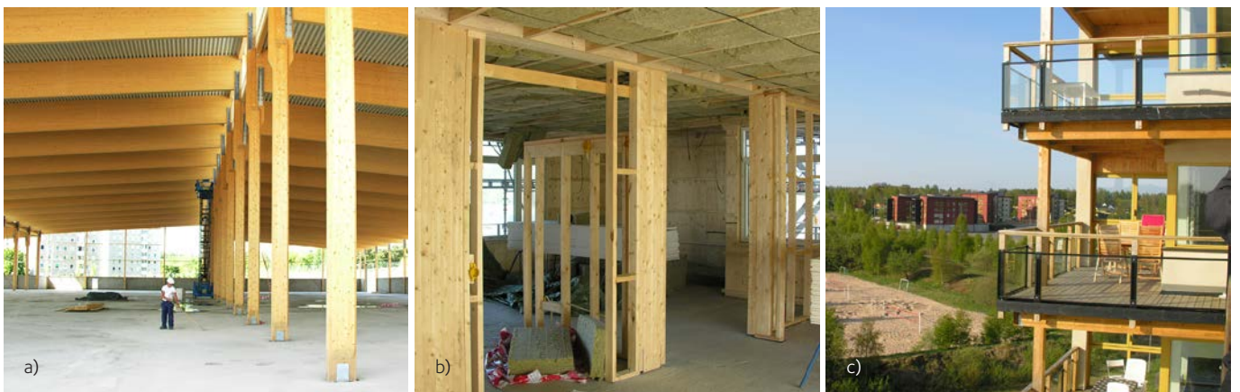
Figure 3.3 Examples of members subjected to compression forces a) Columns in a timber frame, b) studs in a multi-storey timber framed building, c) external columns.
