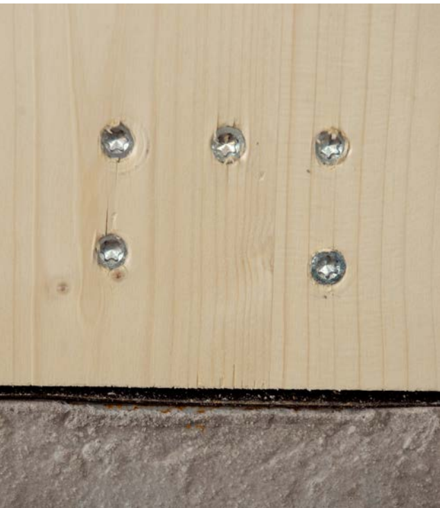
Screwed joint, CLT.
