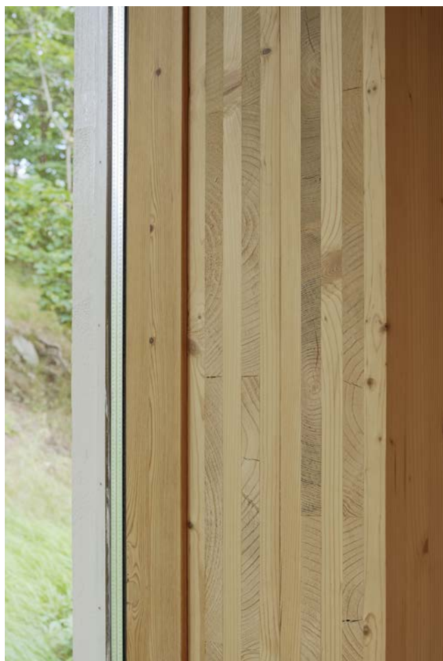
External wall made of CLT.
