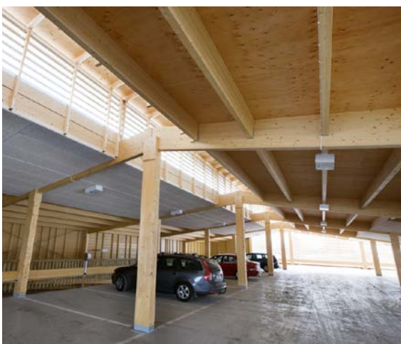
Parking garage with glulam and cross-laminated timber (CLT) frame.
