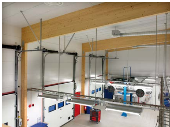
Example of a glulam frame in a car repair shop.
