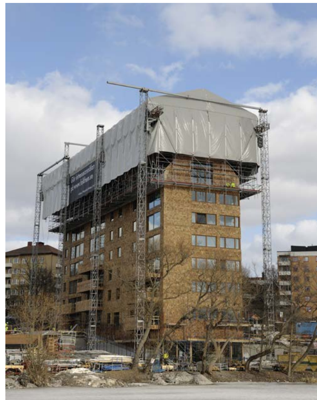
Temporary shelter to protect against the weather when building a timber-framed apartment block.
