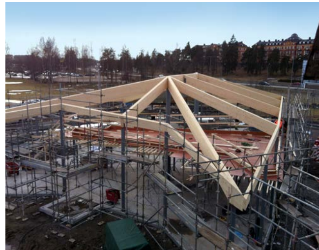
Assembling the glulam roof frame for the Brigade Museum in Karlstad, Sweden.
