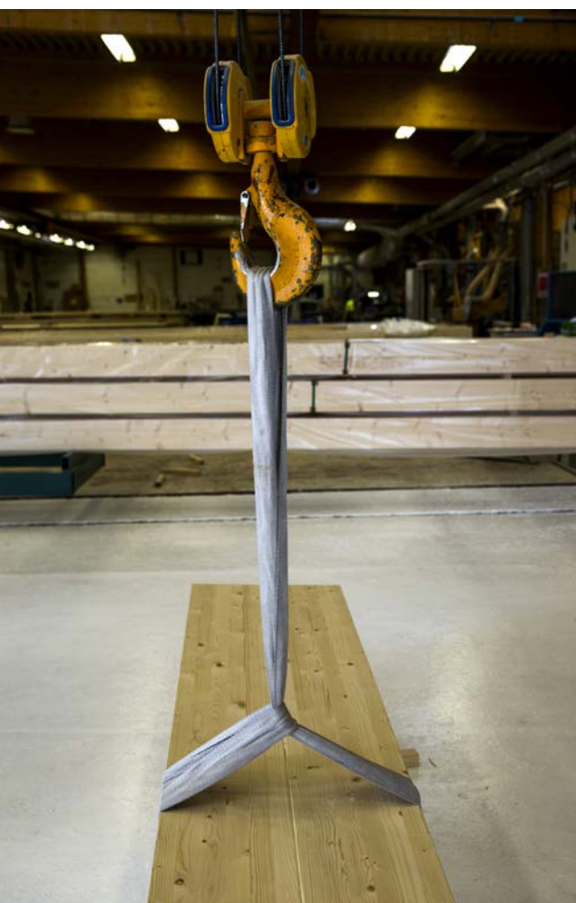
The use of webbing slings avoids edge damage to the glulam element and allows for good balance during the lift. When lifting large, heavy glulam elements, edge protectors should also be used.
