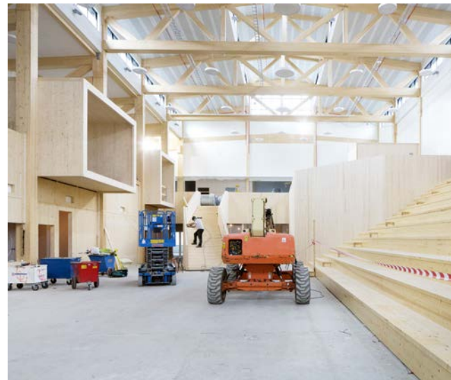
Scissor lift and boom lift during assembly of glulam and CLT frame for school building.
