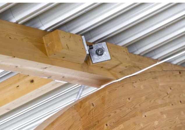
Fixing detail for wind brace in the roof of a glulam frame.
