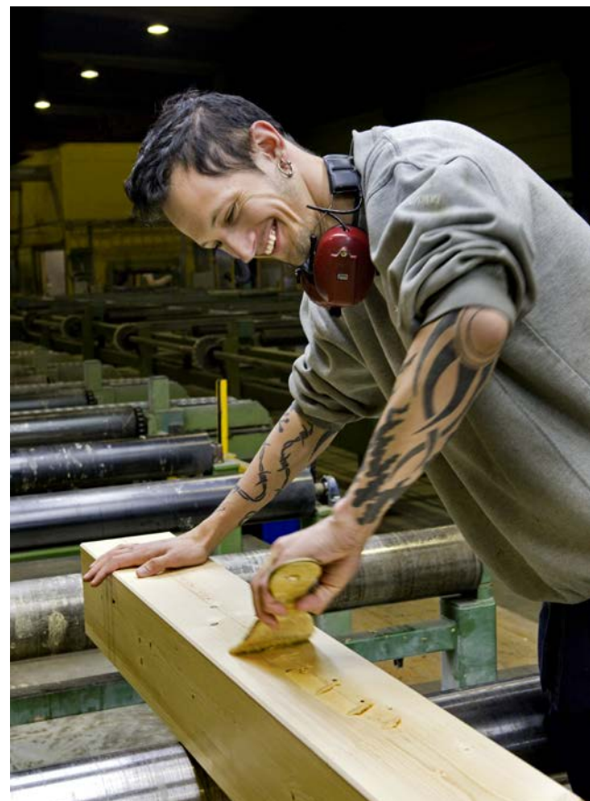
Preparation of a glulam post to be surface treated by the glulam manufacturer.
