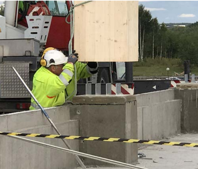
Installing a glulam post with steel plates set into the post shoe.
