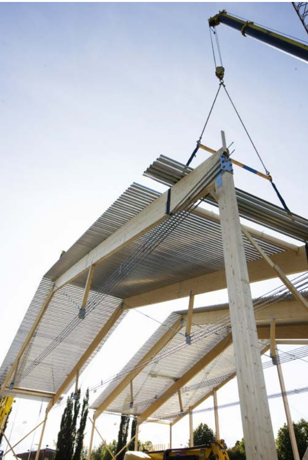
Assembly of three-hinged roof trusses in glulam with steel ties on glulam posts.
