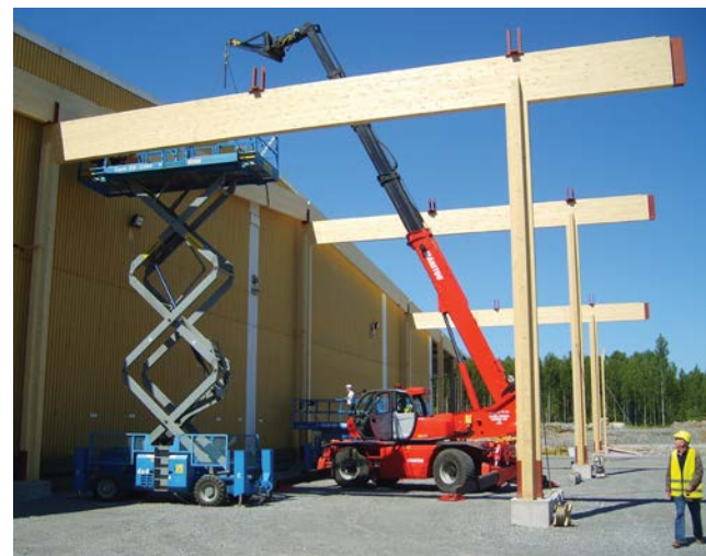
Scissor lift and telehandler used in the assembly of a glulam frame.
