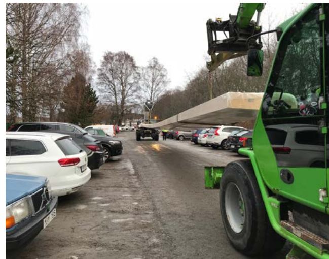
Transporting a long glulam beam with a telehandler on the construction site.
