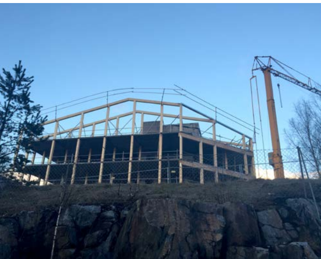
Assembling a storage structure using a truck-mounted crane. Posts and roof beams in glulam, with floor and stairwell in prefabricated concrete.
