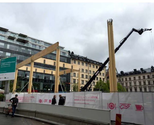
Assembling a timber frame in a dense urban environment. Temporary market hall.
