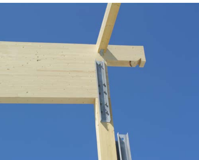
Glulam post-beam connection with UPE steel U-channels and fastening with machine-threaded screws and nuts.
